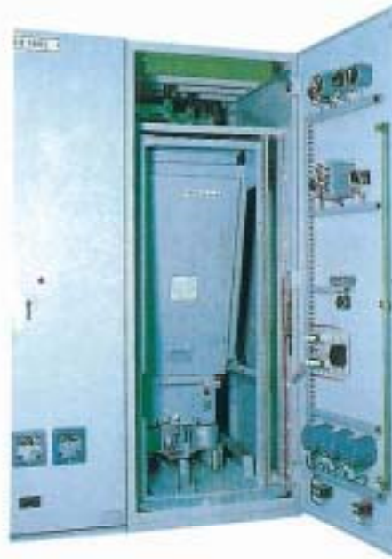
12KV metal-enclosed switchgear
