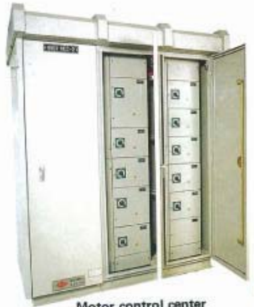
Motor control center (Outdoor type)
