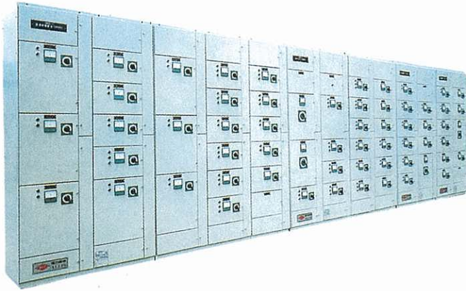
Motor control center (Indoor type)
