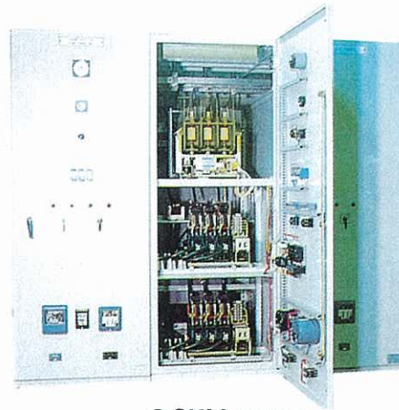
3.3KV motor Starting Panel
