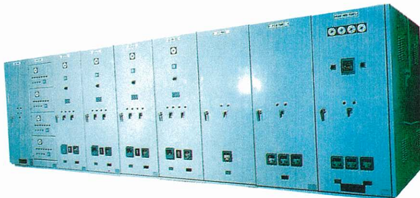
High voltage metal- enclosed switchgear
