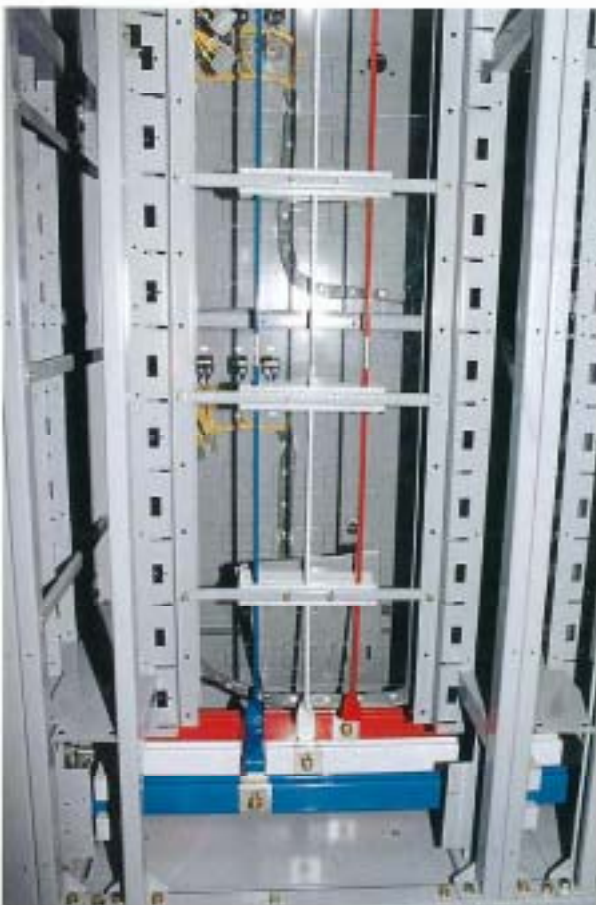
Fig.23 ALLIS BUS BRACE
