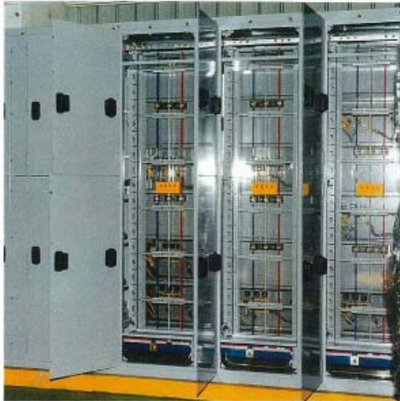
Fig.12 GROUND BUS MOUNTED ON THE TOP
